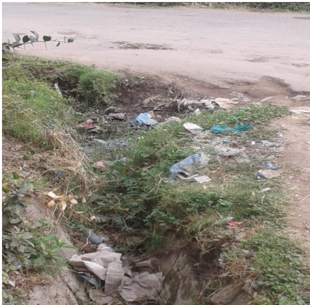
Figure 4-13: Poorly maintained drain at the Junction opposite Uvuvi House Southern gate
