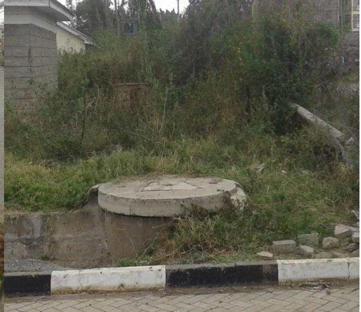
Figure 4-16: Manhole at the southern gate inside the Compound reported to overflow
