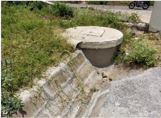
Figure 4-26: NCWSC sewer Manhole on site
