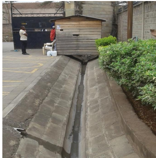
Figure 4-14: A drain from Madina Estate discharging into the drain on Paupau road
